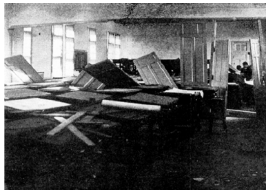
図4 本館2階第二第三製図室間仕切建具の被害 Fig.4 Partition damage of drawing rooms in the second floor of main building.
