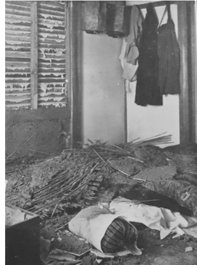
図7 宿直室壁の脱落
