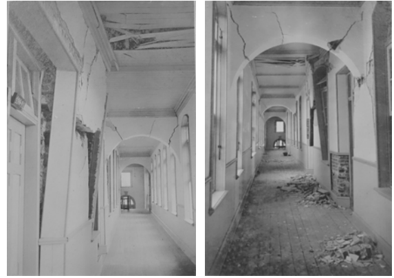
図 15 別館実験棟二階廊下の被害 (左:東より写す 右:西より写す) Fig.15 Damage of corridor in the second floor of annex building.
