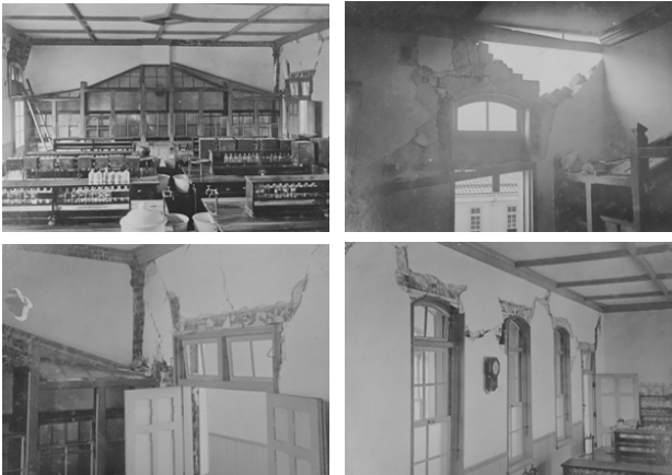
図 12 別館実験棟二階定量分析室の被害 (左上:室仕切 右上:西南隅 左下:西北隅 右下:北側壁) Fig.12 Damage of quantitative analysis room in the second floor of annex building.
