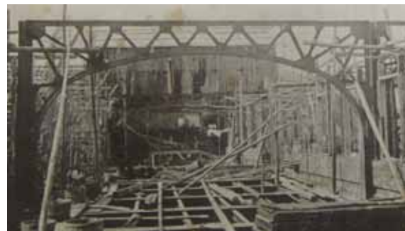
図 22 耐震復旧工事中の別館実験室棟 Fig.22 Repairing of the annex building.
