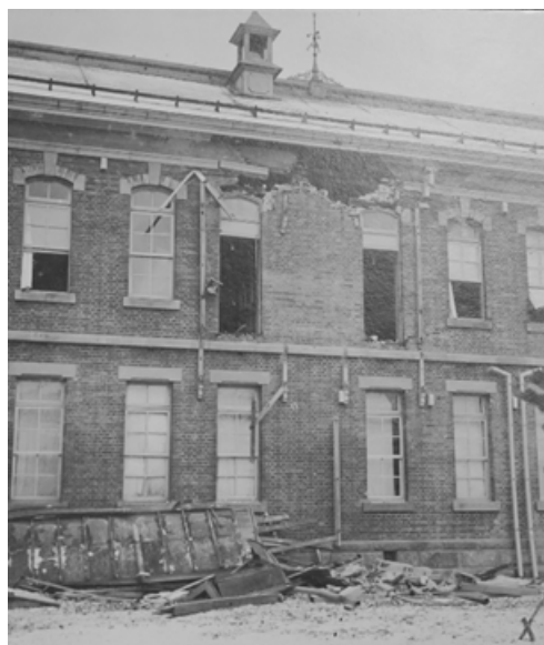
図11 別館実験棟二階硫化水素発生室の破壊脱落 Fig.11 Fallen down hydrogen sulfide generation chamber from the second floor of annex building.
